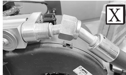
Improperly Seated O-ring Land
