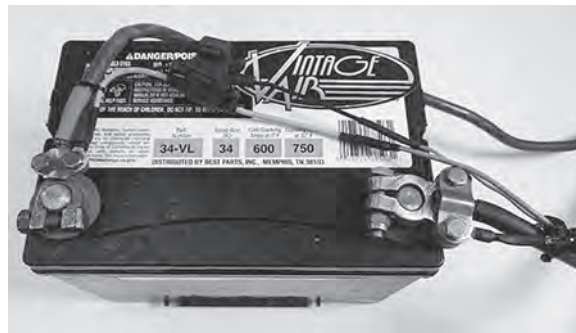
Completed Installation Shown
