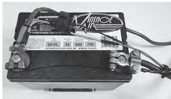
Completed Installation Shown
