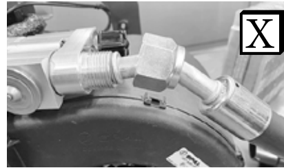
Improperly Seated O-ring Land
