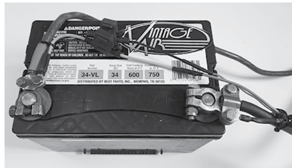
Completed Installation Shown
