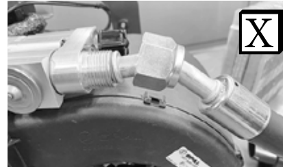
Improperly Seated O-ring Land
