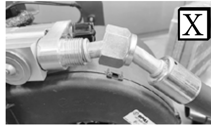
Improperly Seated O-ring Land
