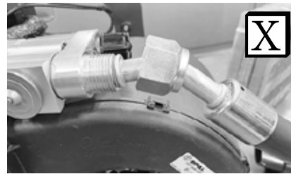
Improperly Seated O-ring Land
